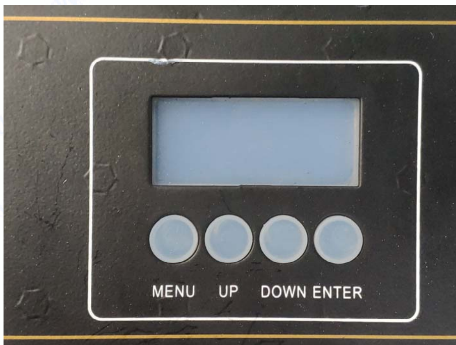
Photo 17: Control panel view
