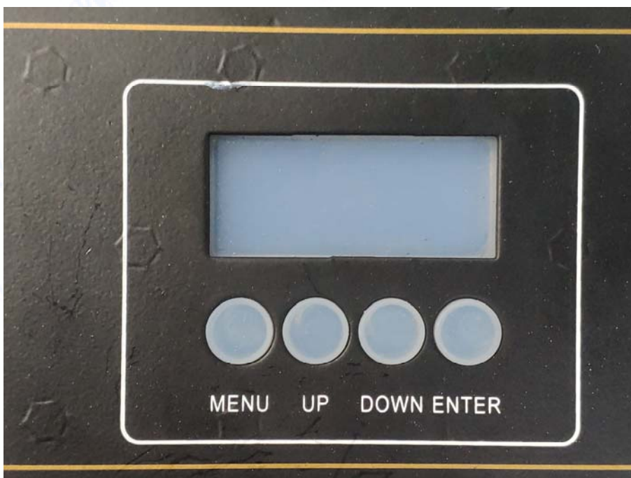
Photo 17: Control panel view
